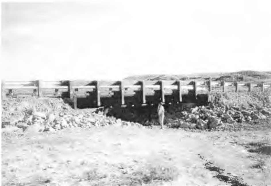
(b) End view of the Cow Gulch Bridge showing the railing system.
