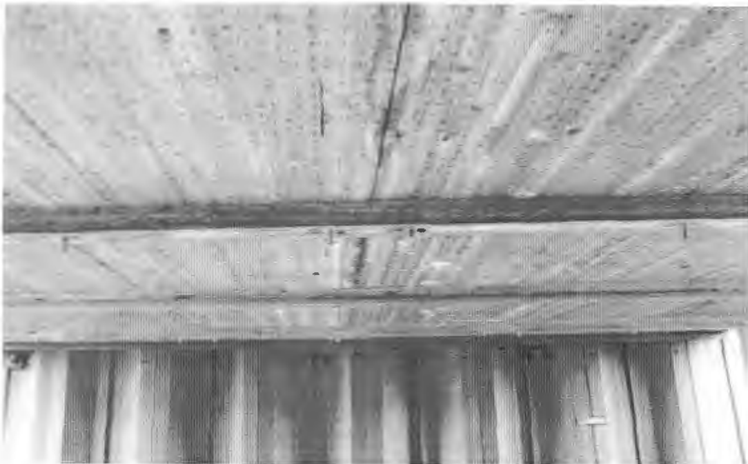
(b) Bottom view showing stiffener beams connected to the deck with thru-bolts.
